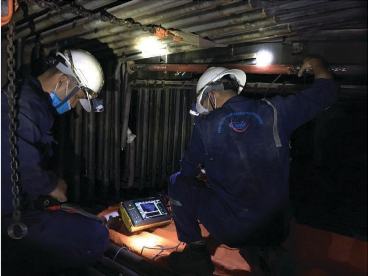
Ultrasonic inspection (Phased Array Ultrasonic Testing -PAUT) of welds after cutting and replacing the boiler pressure pipelines at thermal power plant Nghi Son 1
