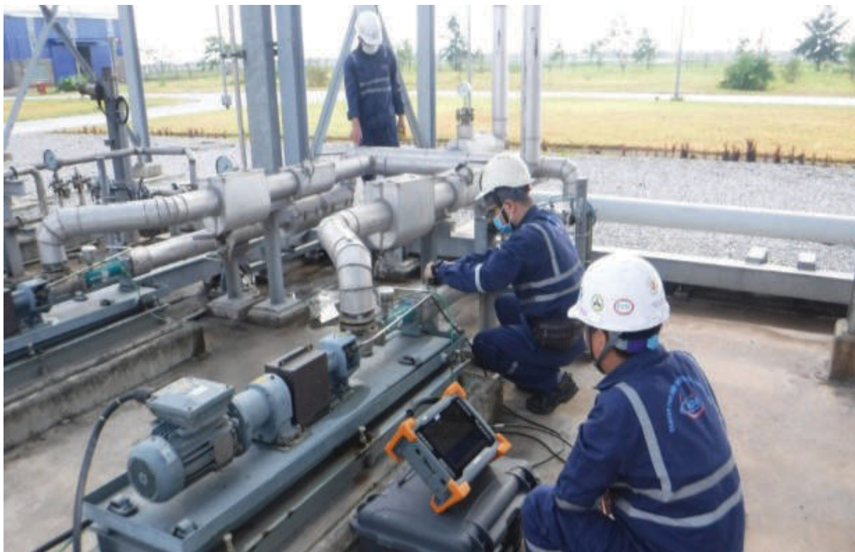
Corrosion testing of pipes at Gas Distribution Center (GDC), Tien Hai District, Thai Binh Province
