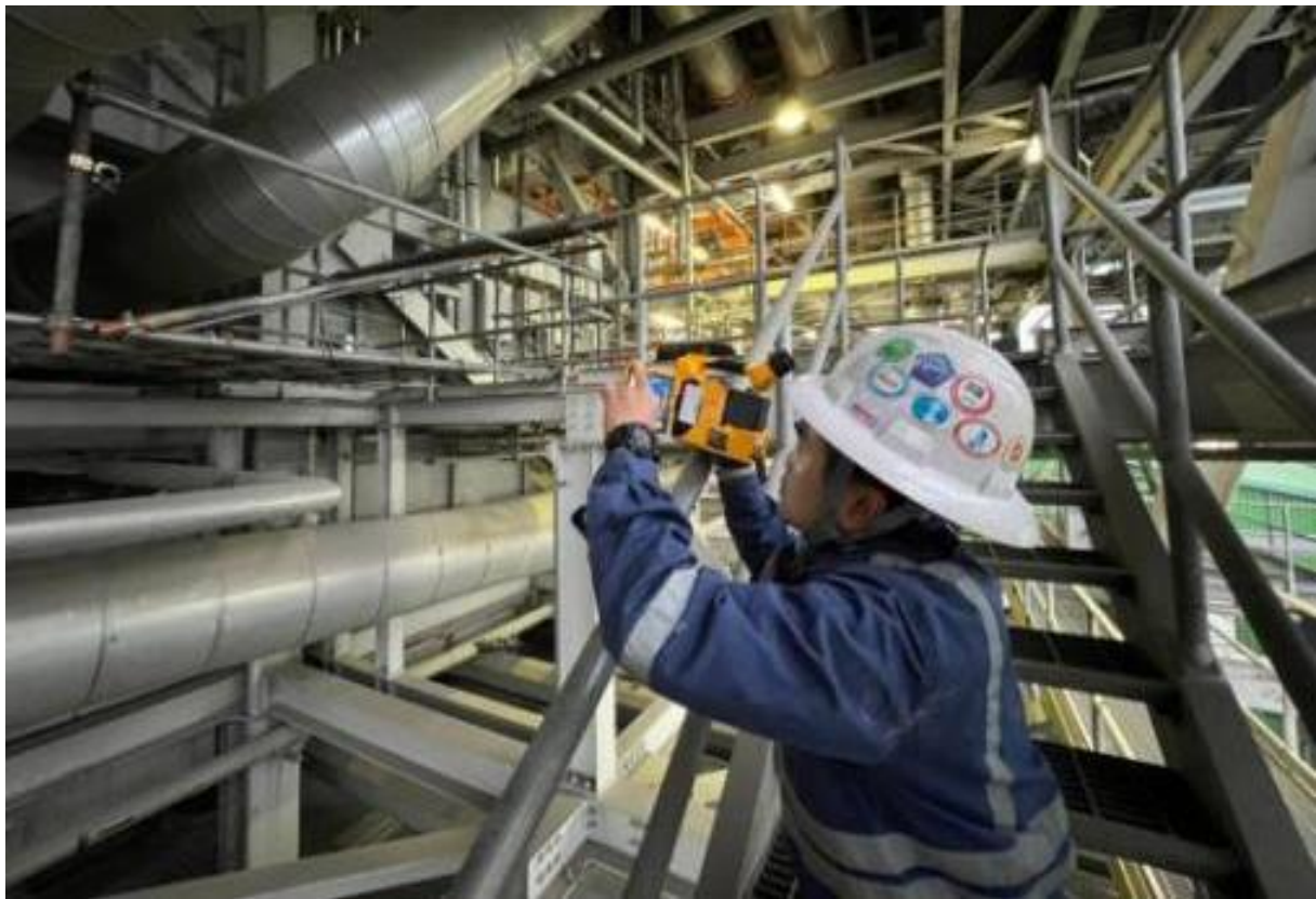
Applying the NDT inspection program at Nghi Son 1 thermal power plant under ministry-level projects 2021-2023
