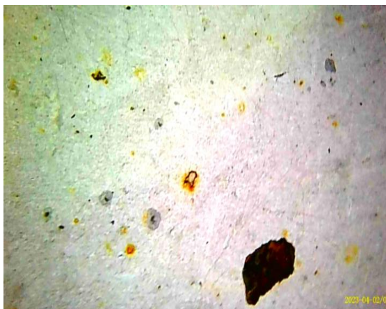
2a. Corrosion hole on beam tube No. 3
