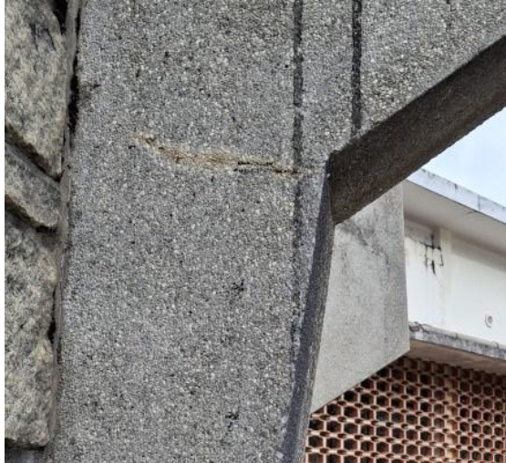
3a. Cracks on the concrete column
